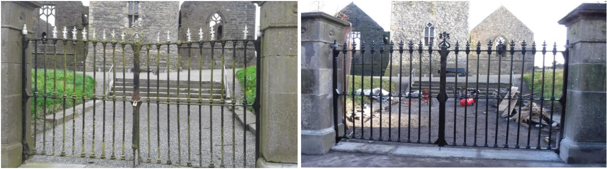
Before and After images of works to 19 th century wrought iron gates, St. Mary's Church Callan.
