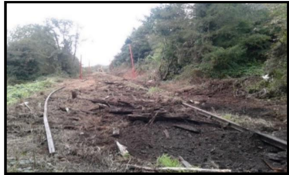
Lifting of old rails and sleepers along the route of the South East Greenway
