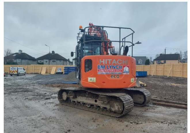
Works have commenced on 22 Part V and Turnkey Apartments at Marnellsmeadows, Callan Road, Kilkenny City
