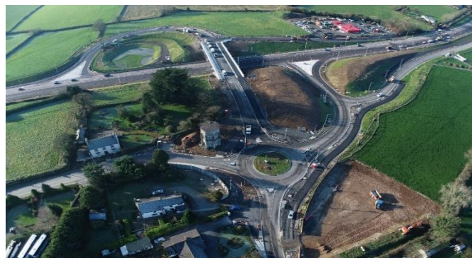
Overhead drone footage of the compacted grade separated junction under construction (N24)
